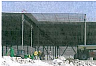
Workers start building the walls that will surround the 677,088-square-foot warehouse that's going up in Lehigh Valley Industrial Park VII, near Route 412 in Bethlehem.
